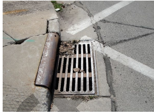
Parallel bar grates can be hazardous to bicyclists.
